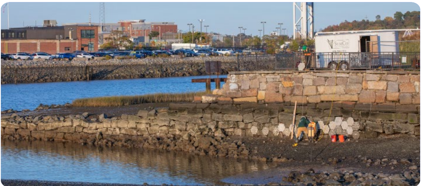
A living sea wall is installed at Condor Street Urban Wild in East Boston. Photo © Sindayiganza Photography
